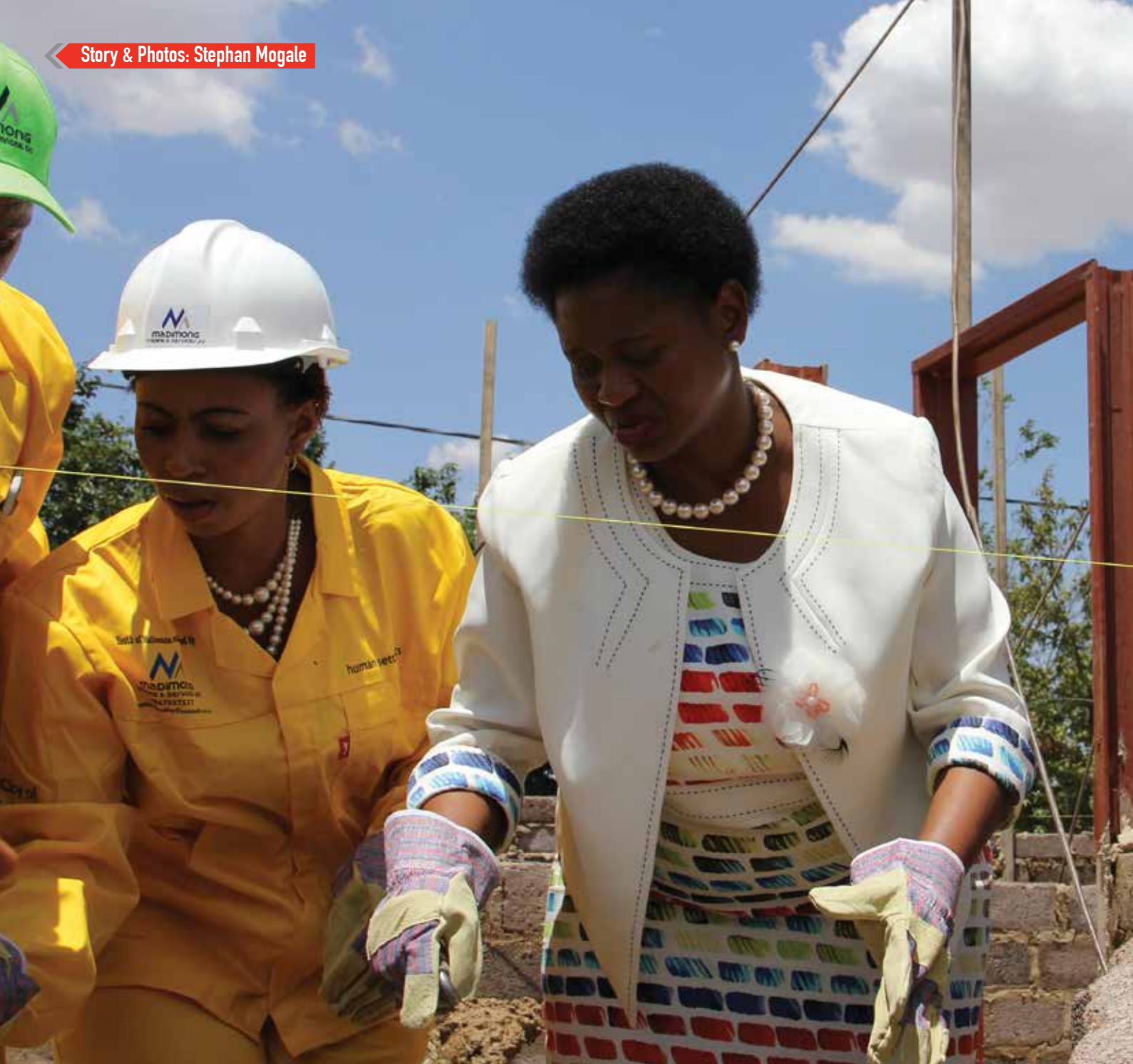
Deputy Minister Zou Kota-Fredericks with Cllr Mampho Thelejane laying bricks in Kanana
