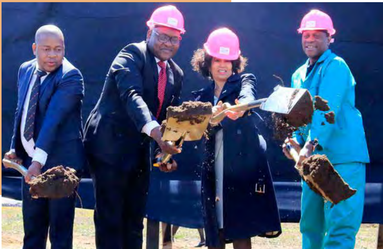
During the sod turning of John Dube City project from left: Mayor of Ekurhuleni Mzwandile Masina, Premier of Gauteng David Makhura, former Minister of Human Settlements Lindiwe Sisulu and former Gauteng MEC of Human Settlements Paul Mashatile
